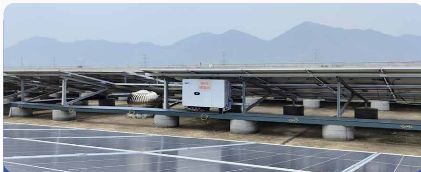
5.916MW Rooftop PV Plant in Hubei, China (XG100KTR, XG50KTR)
