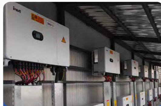
2MW Rooftop PV Plant in Türkiye (XG110KTR)
