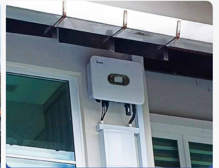
12kW Solar System in Malaysia (XG12KTR)
