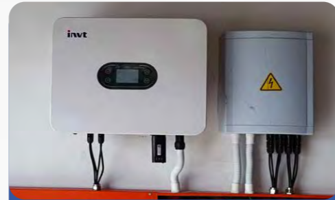
25kW Solar System in Malaysia (XG25KTR)
