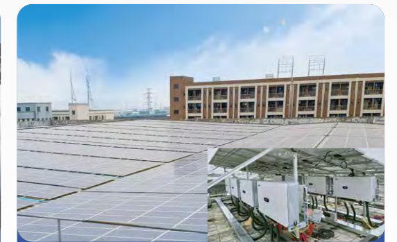
1.1MW Rooftop PV Plant in Guangdong, China (XG110KTR, XG30KTR)
