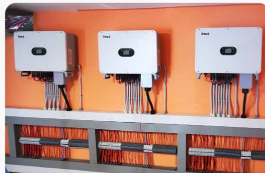
180kW Rooftop PV Plant in Lebanon (XG60KTR)
