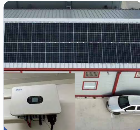
25kW Solar System in Slovakia (XG25KTR)
