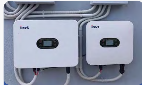
16kW Solar System in Greece (XG6KTL, XG10KTR)
