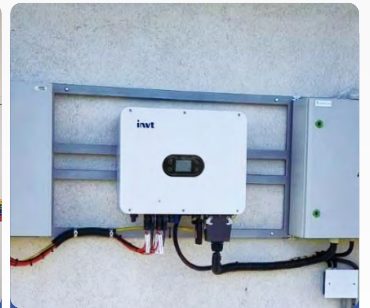
30kW Solar System in Serbia (XG30KTR)
