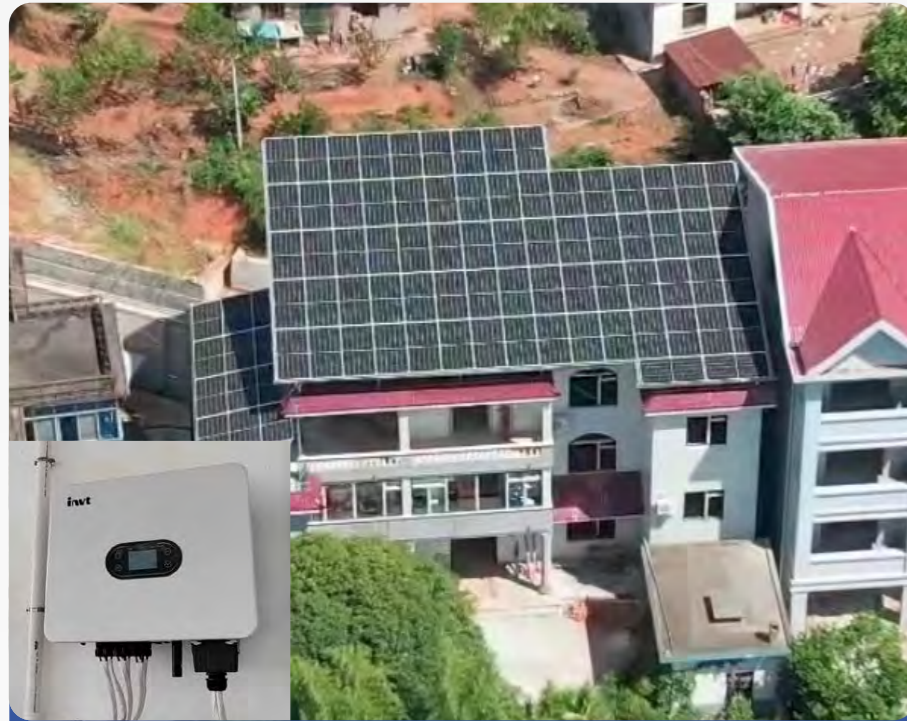
40kW Solar System in Jiangxi, China (XG40KTR)
