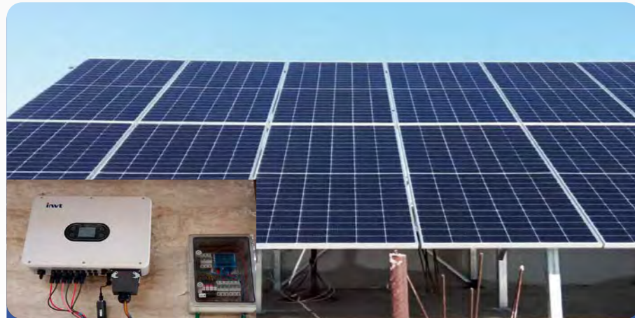
30kW Solar System in Israel (XG30KTR)
