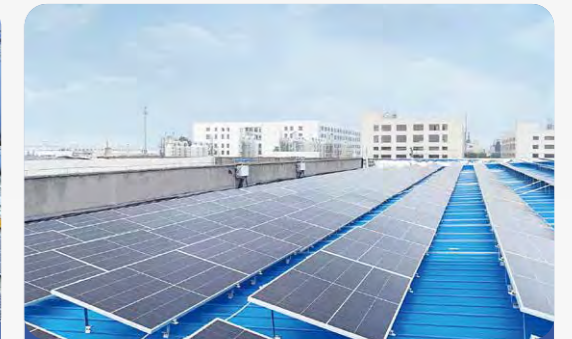
1.2MW Rooftop PV Plant in Jiangsu, China (XG100KTR)
