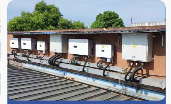
522kW Rooftop PV Plant in Zhejiang, China (XG110KTR, XG60KTR, XG50KTR)
