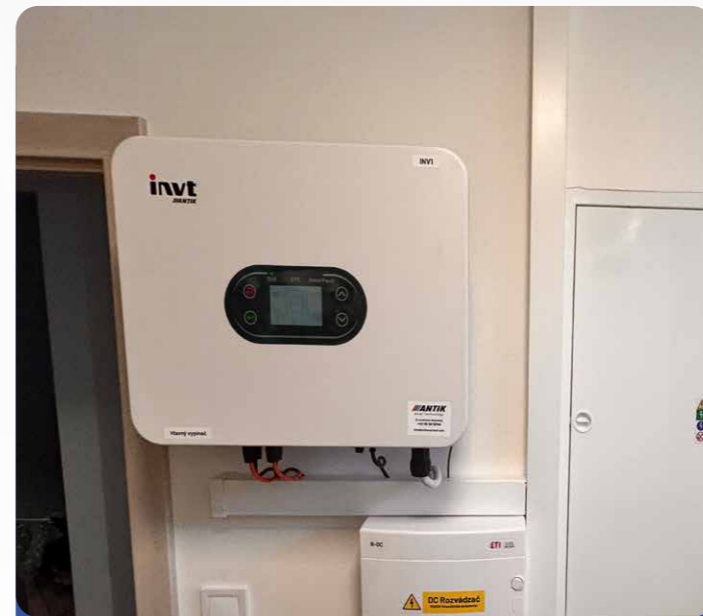
10kW Solar System in Slovakia (XG10KTR)
